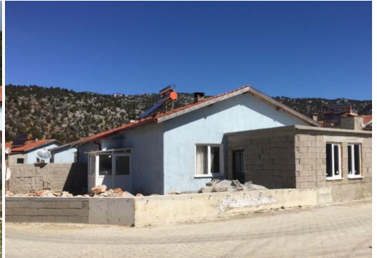
Figure 9. House with the frames replaced and an entrance unit and bakery added
