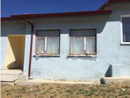
Figure 12. Measures taken by the residents in the windows against the water ingress problem
